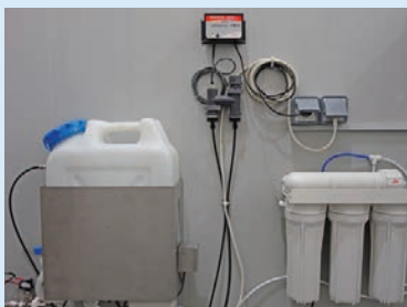
Water treatment systems
