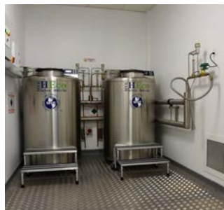
CryoRoom Design & Installations
