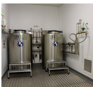
CryoRoom Design & Installations
